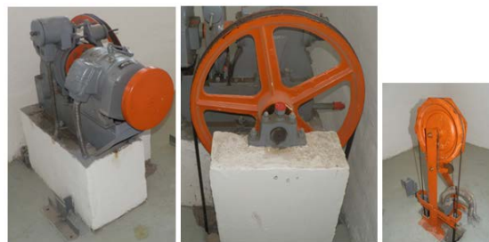
Fig. 3 Elevator machinery, traction wheel and speed-limiter
