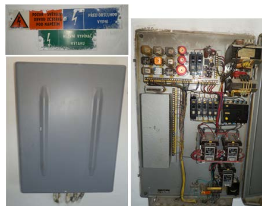
Fig. 4 Electric installation of the lift
