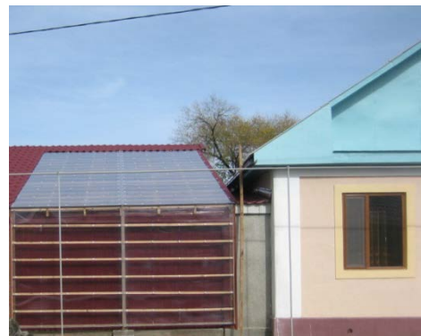
Picture 2 - The experimental module of thermal point attached to the rural house
