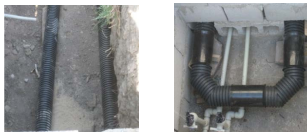
a - trench with the heat exchange pipe; б - the heat exchange pipe in the viewing hole
