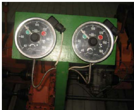
Figure 9. Devices for measuring and controlling the gearbox oil temperature
