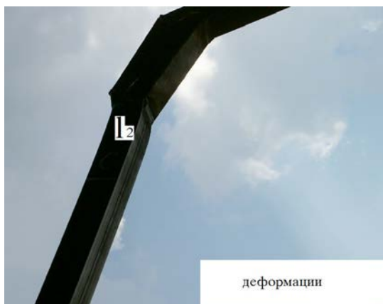
Fig. 4: Deformations on link between vertical and roof tube
