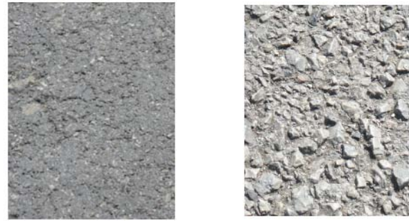
Fig. 4 The tested road surfaces; left: asphalt-concrete smoothed (ACS); right: asphalt-concrete roughened (ACR).
