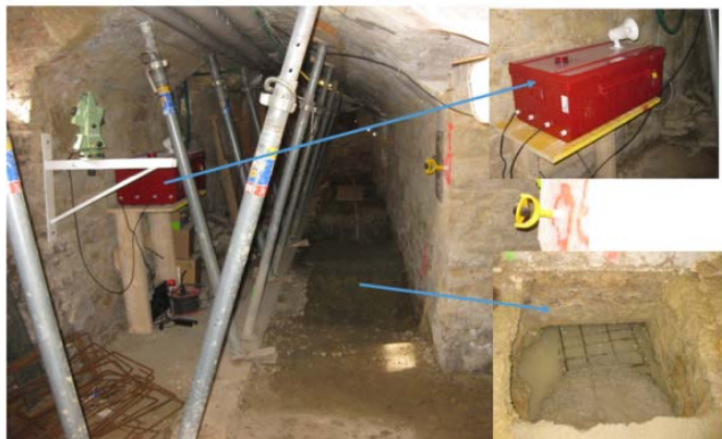
Fig.5. Gauging station and signaling points
