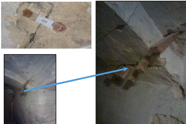
Fig.2. Cracks in the basement wall
